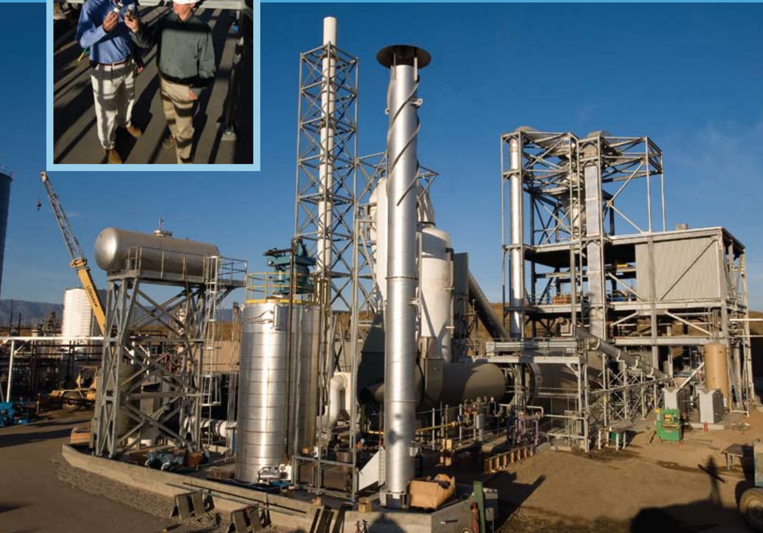
Dryer Area, Rialto Biosolids Processing Facility, CA
